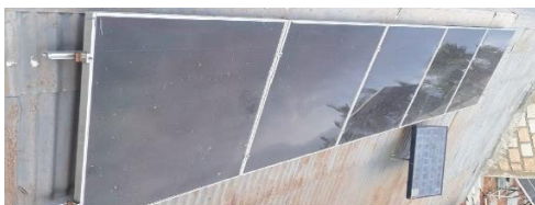
Gambar 6 Hasil Instalasi Sistem Rooftop On Grid
